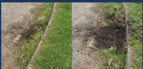
Ridgeway Crescent, Whitchurch Gully Uncovered
